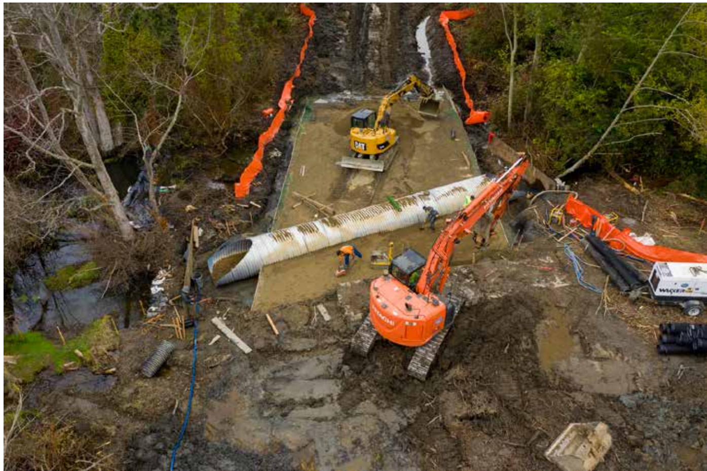
Work continues this week at Clallam County's Lower Dungeness Floodplain Restoration Project as workers with Scarsella Brothers install a new culvert in Meadowbrook Creek, a tributary to the Dungeness River. The ecosystem restoration effort includes setting back a portion of the Dungeness Levee to offer greatly improved flood protection while restoring acres of lost floodplain needed as habitat for endangered salmon, according to project manager Cathy Lear of the Clallam County Department of Community Development. Project funding comes from Floodplains by Design and the Puget Sound Partnership's Puget Sound Acquisition and Restoration Program. The project is identified in the Puget Sound Chinook Recovery Plan. Dungeness Chinook population must be recovered in order for endangered Puget Sound Chinook to be delisted. Photo by John Gussman
