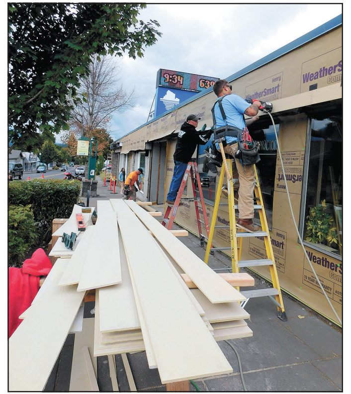
Jared Eck, left, Joe Kovacs and Larry Bosckis with RSV Building Solutions of Vancouver install new siding at the Riverview Community Bank in Stevenson on Friday, Aug. 27. The bank is being renovated inside and out. Photo by Philip L. Watness
