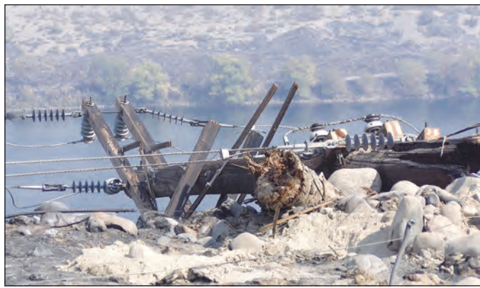
Douglas County Public Utility District Damaged electrical equipment sits on the Douglas County side of the Columbia River.
