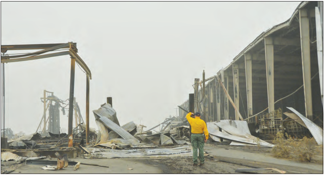
AL CAMP | Special to The Chronicle A visitor with Commissioner of Public Lands Hilary Franz surveys damage to the former Omak Wood Products Mill. Rodney Cawston, Colville Business Council chairman at the time, said he hopes the mill and the Malott HUD housing site, where several homes were lost, will qualify for FEMA funding. With all the destruction — public, private and the loss of life — “I don't think people realized how much was burned,” he said.
