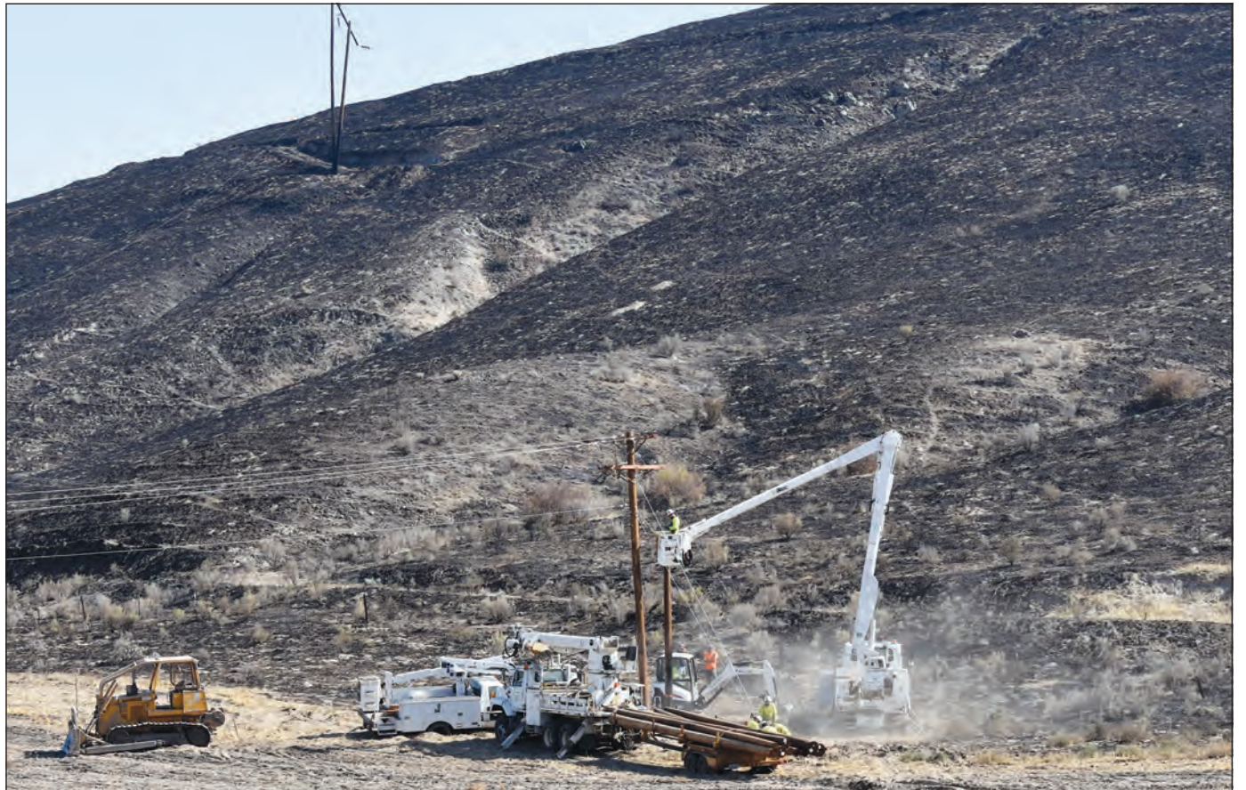
An Okanogan County Public Utility District crew works on replacing damaged electrical lines off Cameron Lake Road.
