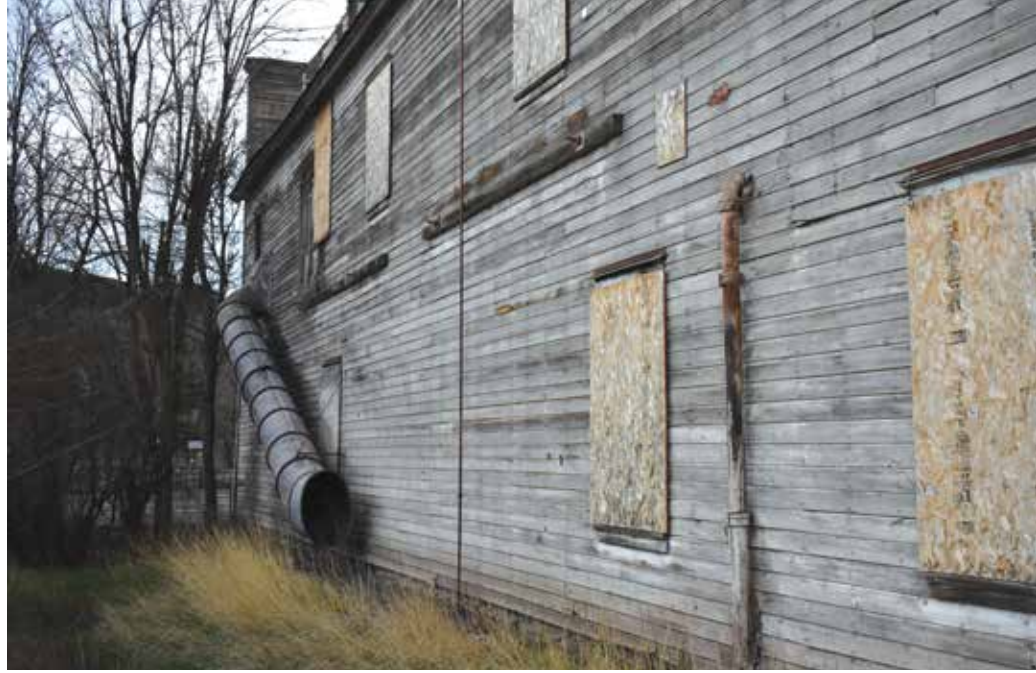
Since acquiring the Lodge property in 2018, the Washtucna Heritage Museum board has mothballed the building. There is still a lot of work to be done on it. Rebecca Pettingill photo
