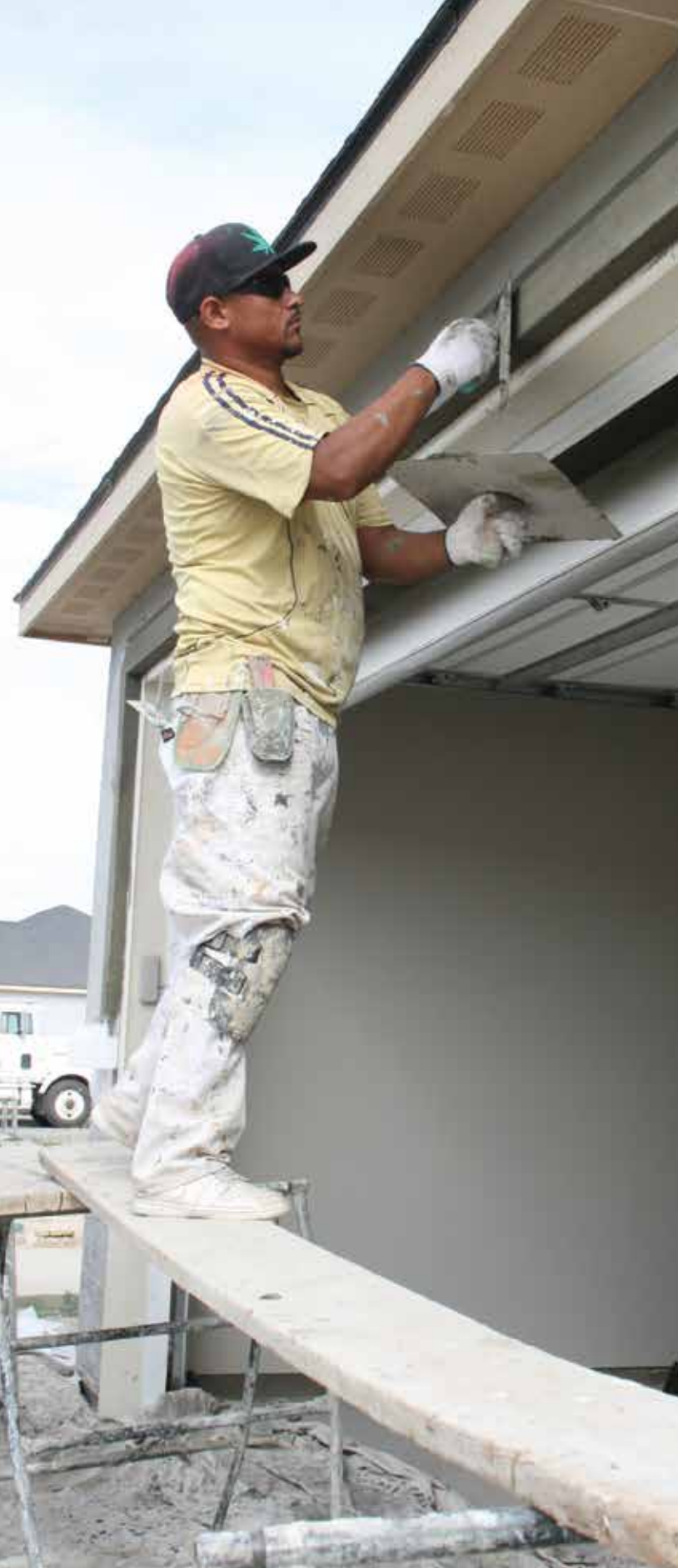
Sergio Infante works on the garage of a house under construction in Othello in 2021. City officials are working on revisions to the city's building regulations to make it easier to build in town. File photo
